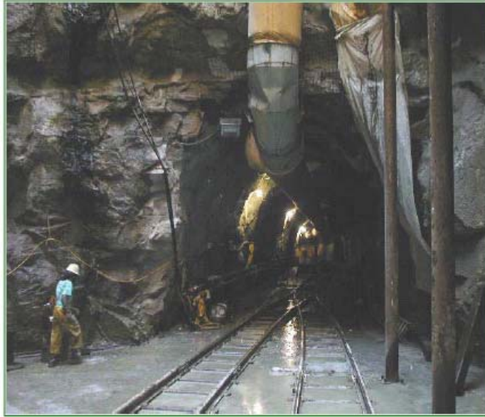
Figure 3. Starter Shaft for Deep Tunnel Construction between Richmond CSO 4 and CSO 5 (Chandler et al., 2003).
