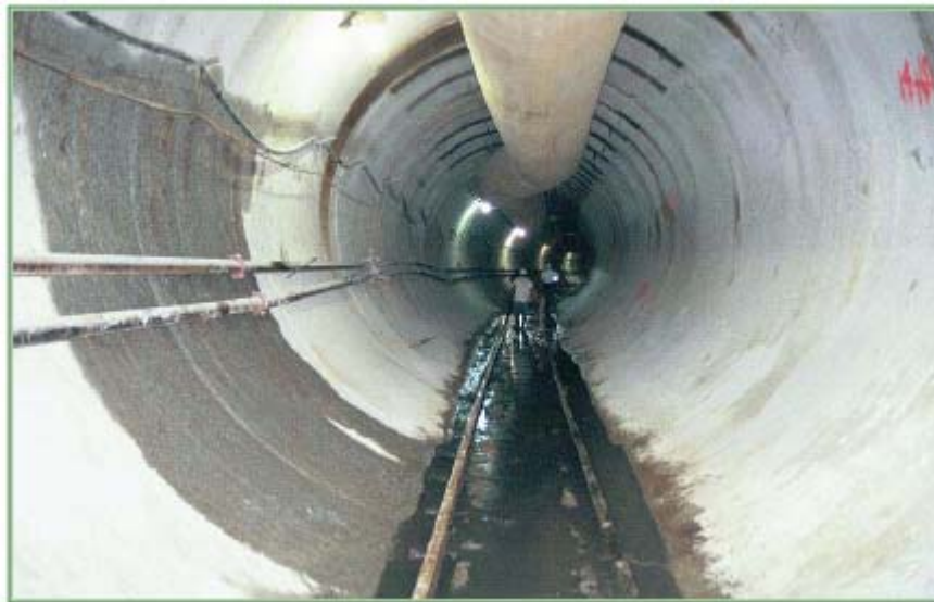
Figure 4. Rock conditions in the Tunnel Shaft between Richmond CSO 4 and CSO 5 (Chandler et al., 2003).
