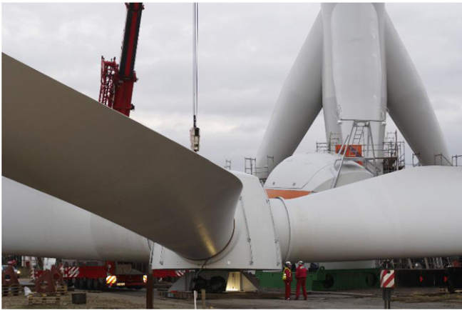
Figure 16. An offshore wind turbine with tripod is under construction. Note that the tripod design is different to the one shown in figure 15 in order to lower the stress at the joints.
