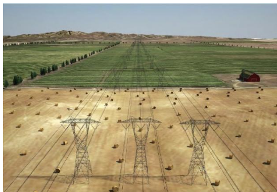
Three 500 kV lines 600 foot ROW
