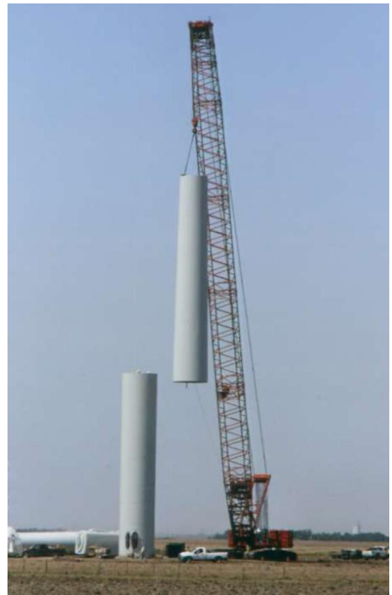
Figure 1.1: Tubular Steel Tower (Courtesy of T. Baird, Iowa State University)
