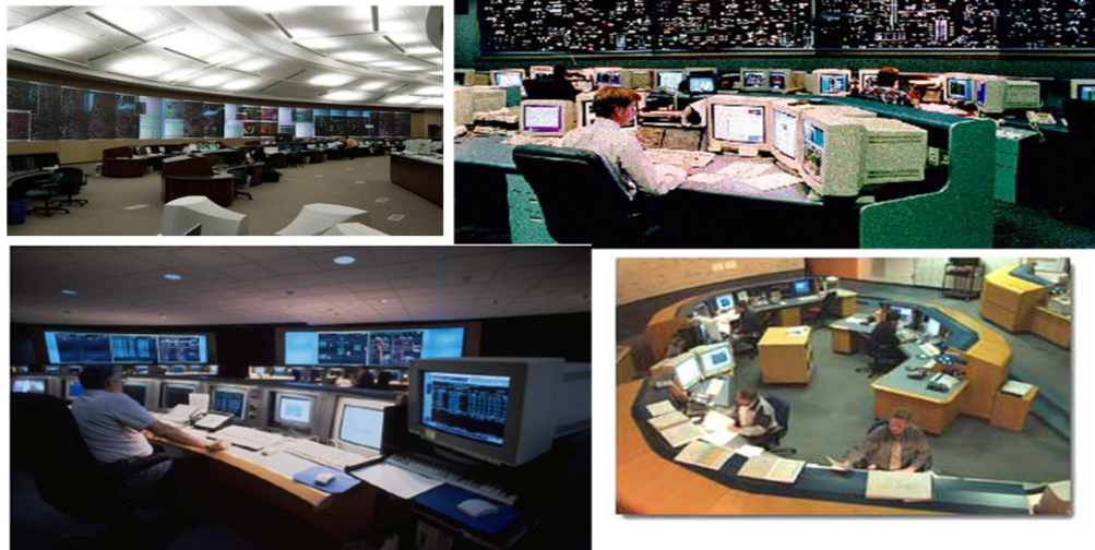
Fig 0.d: Energy control centers
