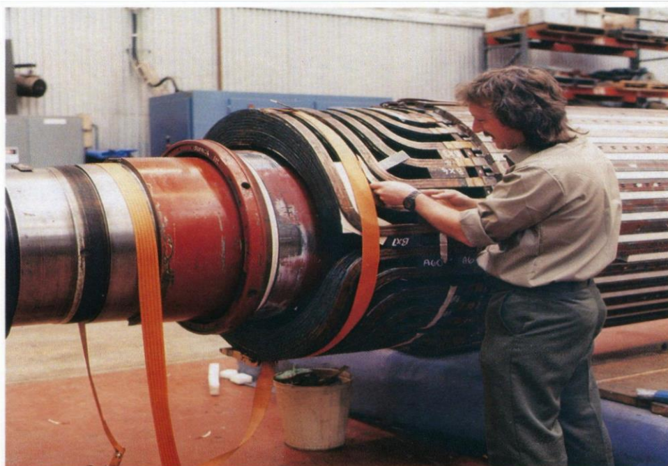
Repairs to the overhand insulation of this 200MW generator rotor were carried out by experienced tradesmen working on shift to ensure the earliest possible return to service.
